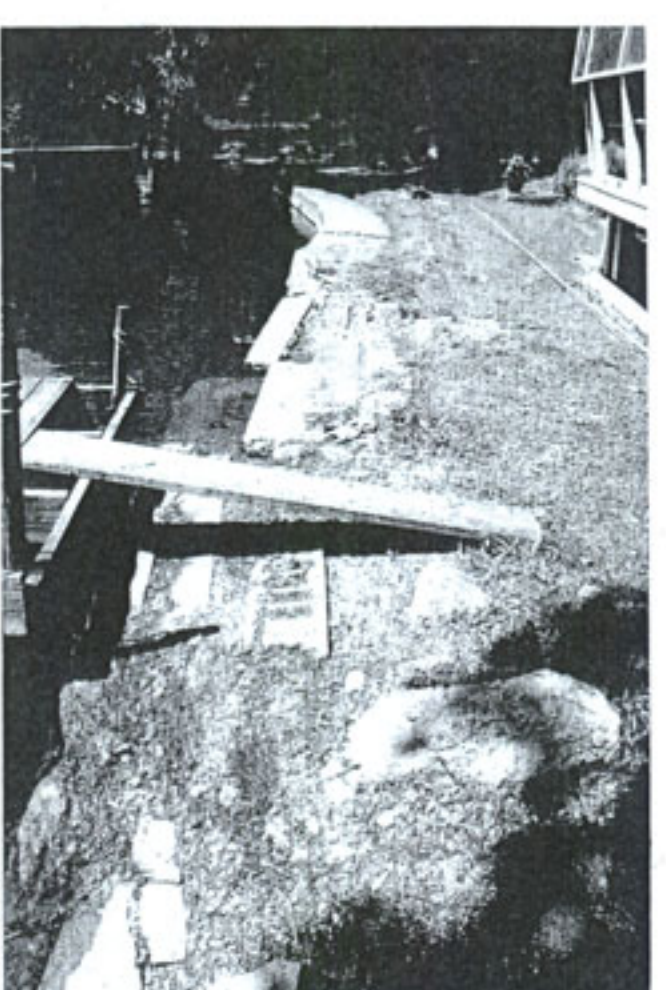
Photo E Flooding and winter ice damage
